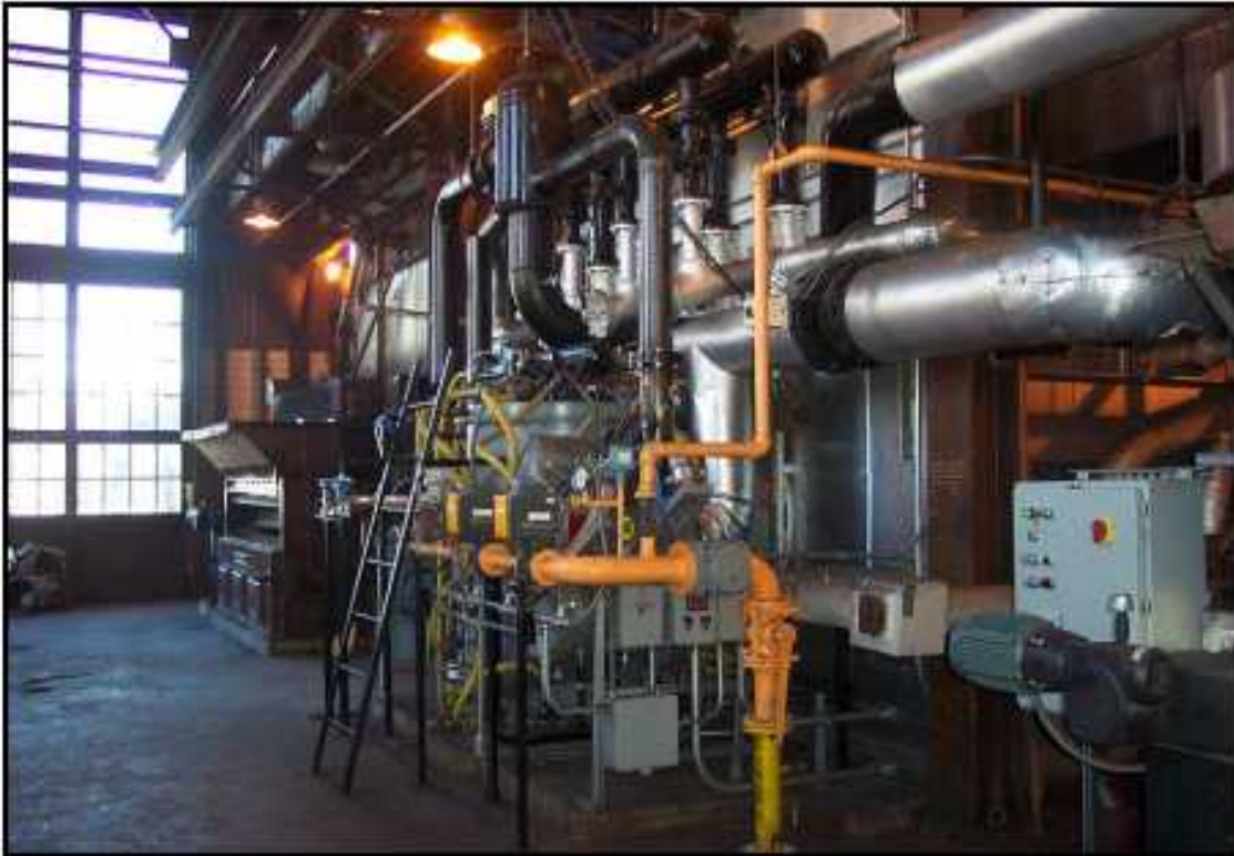
Figure 8. Ashworth ( 40 \times 10^6 Btu/hr) Gasifier-Combustor System.
