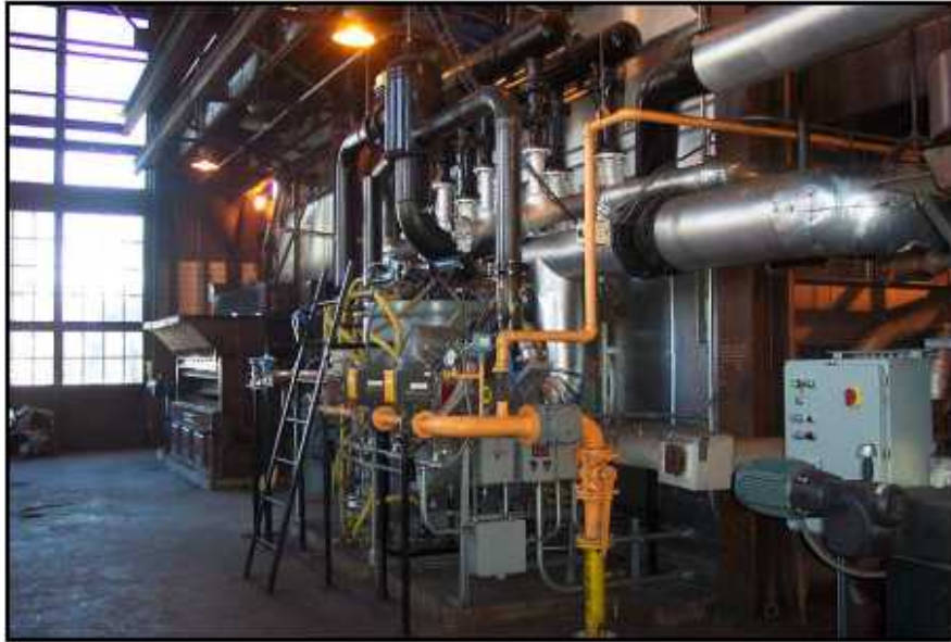
Figure 7. Ashworth 40 x 10 6 Btu/hr 3-Stage Combustion System.
