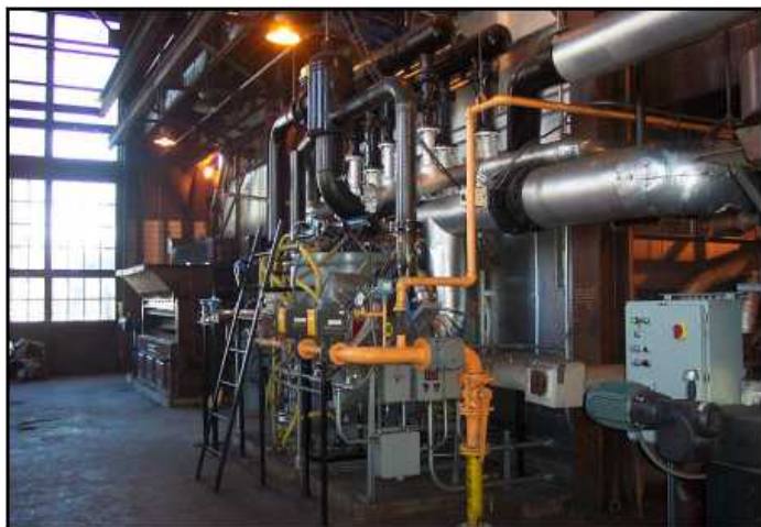
Ashworth Gasifier - Combustor
