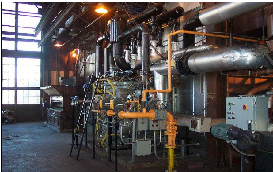
Figure 6. Ashworth 40 \times 10^6 Btu/hr 3-Stage Combustion System.
