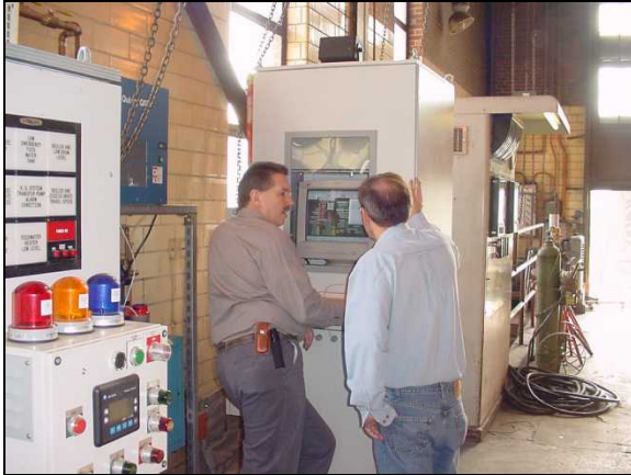
Figure 9a. Allen Bradley and DeltaV Control.
