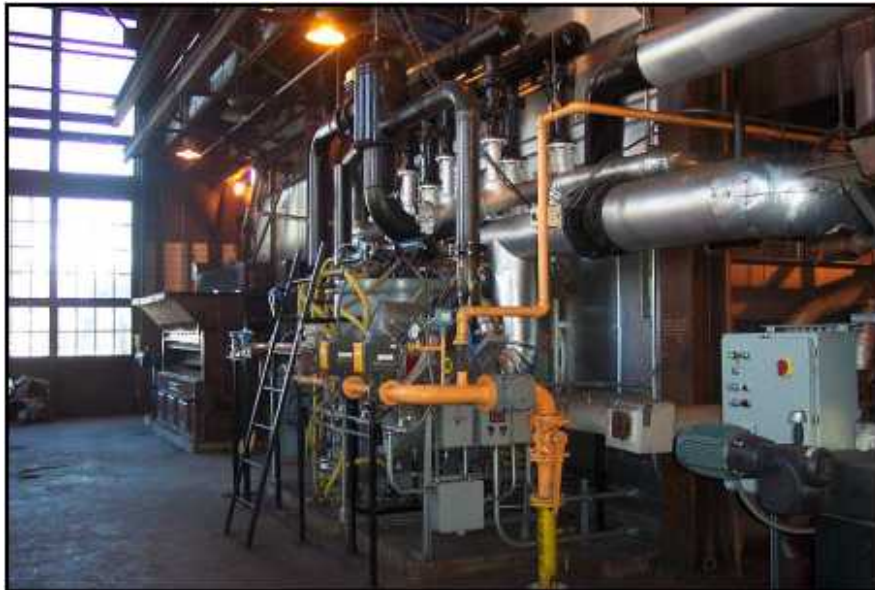
Figure 7. Ashworth 40 x 10 6 Btu/hr 3-Stage Combustion System.
