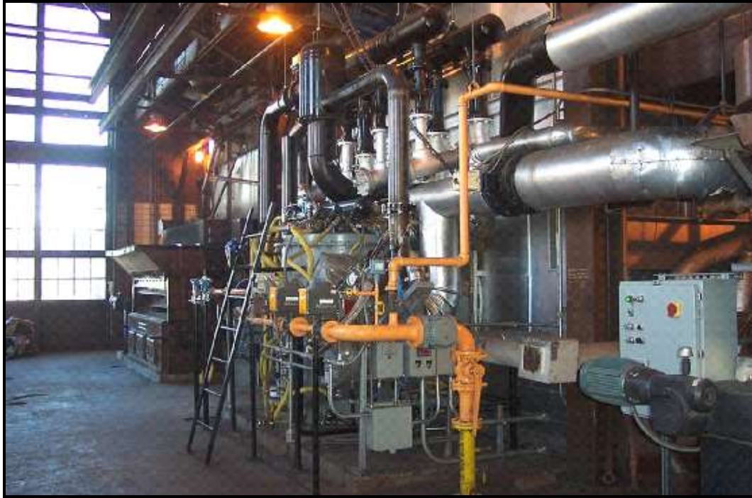
Figure 5. Ashworth (40 Million Btu/hr) Gasifier-Combustor System at Lincoln.
